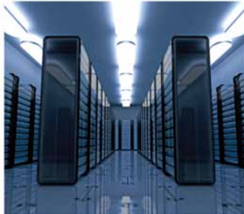
Racks of servers at a data center.
